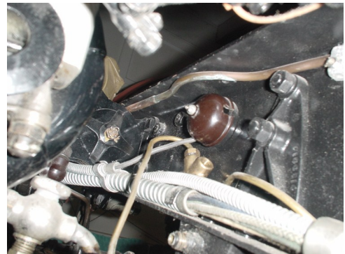
FF-6 Horn Wire Junction Box
